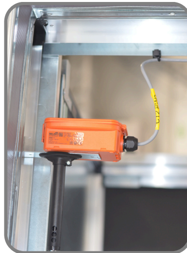
Installed automation control and measurement elements
