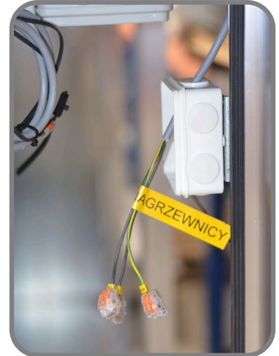
Signal to the valve actuator derived near the exchanger stubs
